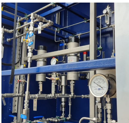
Completed unit prior to mobilisation
