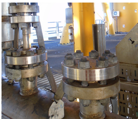
Incumbent flanged connection system.
