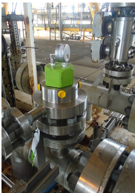
Replacement chemical injection access fitting.
