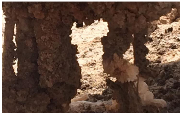
Large build up of scaling on underside of pipework
