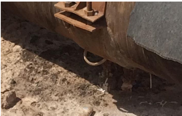
Live leaking defect found at the 6 o'clock position
