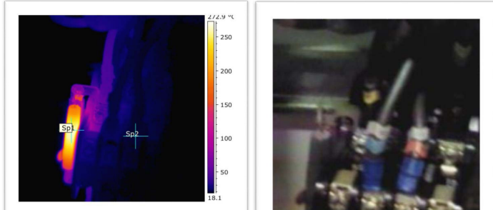
Resistor displaying temperature of 250 degrees which is significantly above ambient and operating temperature. This was classed as a serious priority.
